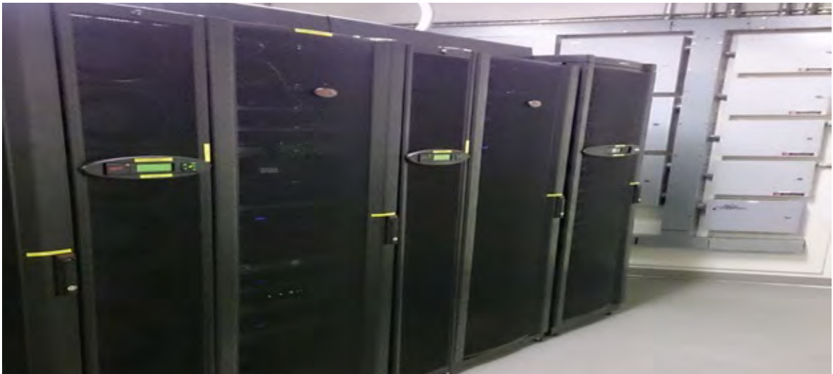
Networking and data storage equipment
