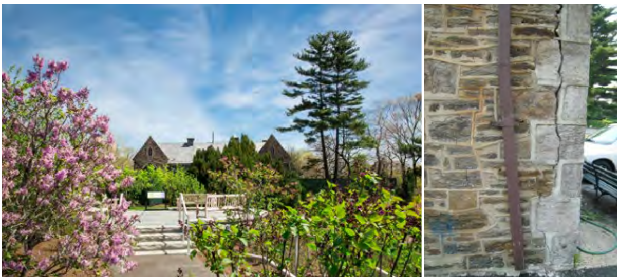
A historic structure in dire need of repair and renovation
